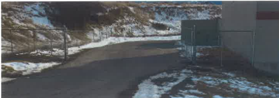
New gate and the chain link fence moved back for easier access for delivery trucks.
